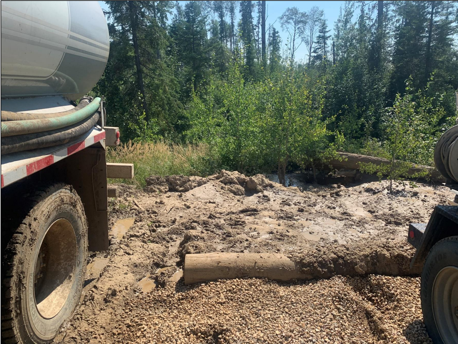
Photo 01: Hydrovac Waste Point of Release
