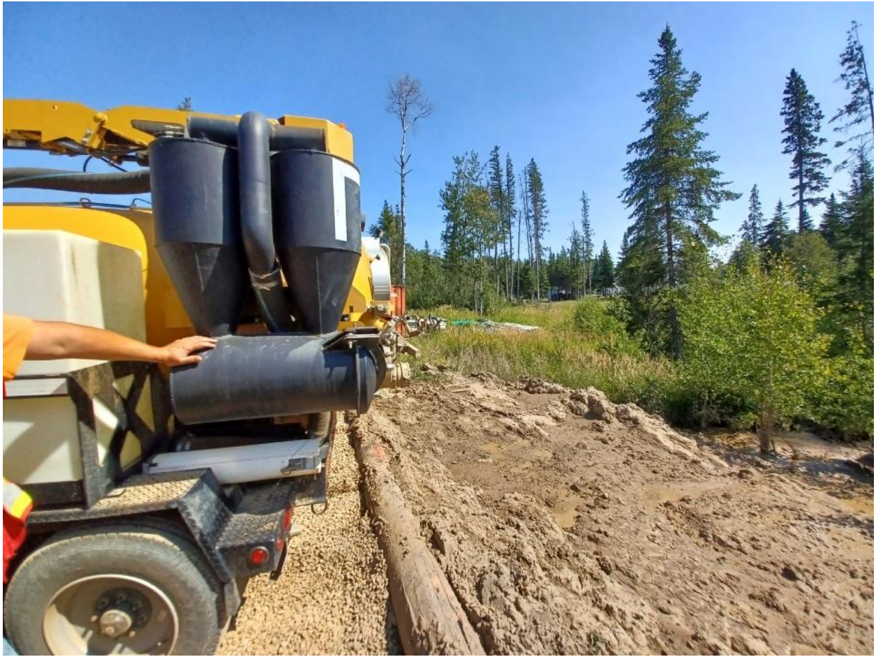
18. Heavy Equipment, Grading Alterations and Contaminant Discharge Concern
