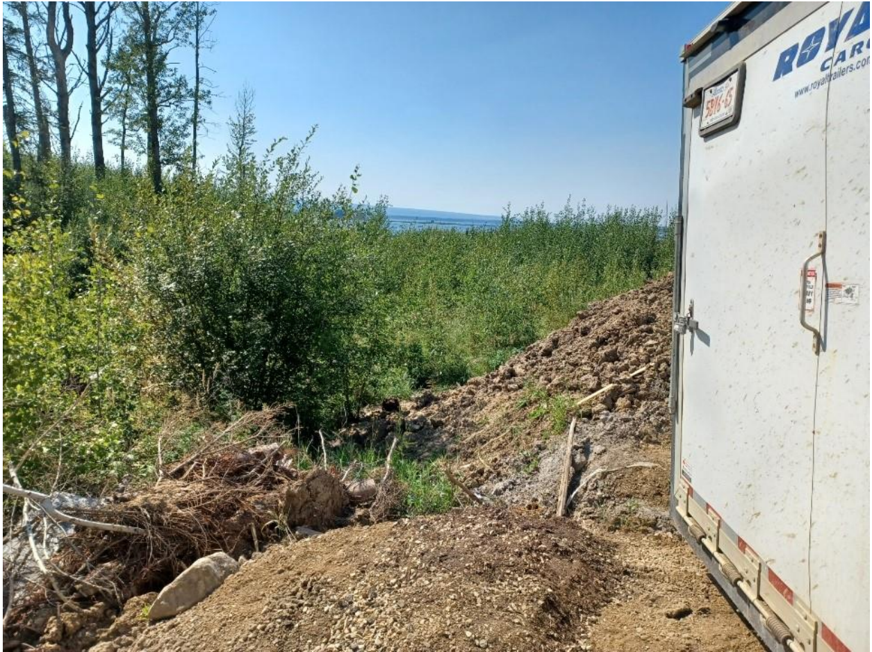
10. Heavy Equipment, Storage, Environmental Reserve Encroachment, Excavation and Grading Alterations
