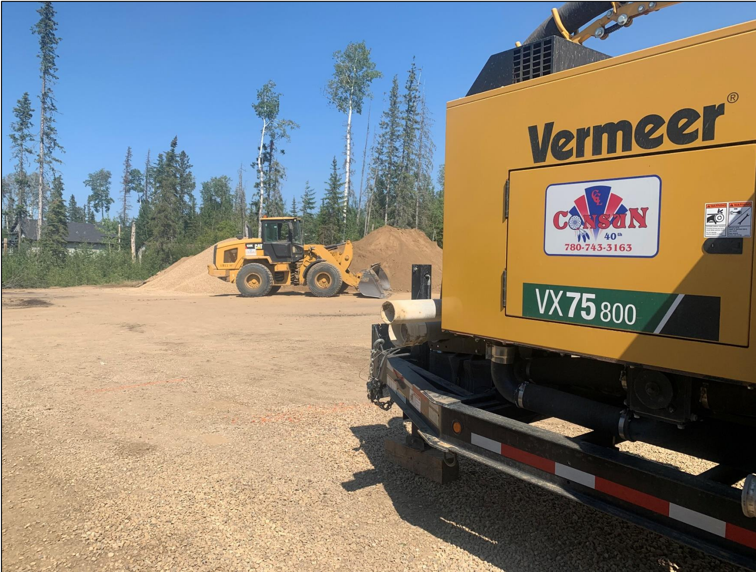
Photo 05: Onsite Equipment at the Laydown Yard
