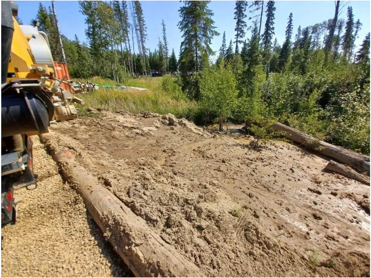
19. Heavy Equipment, Grading Alterations and Contaminant Discharge Concern
